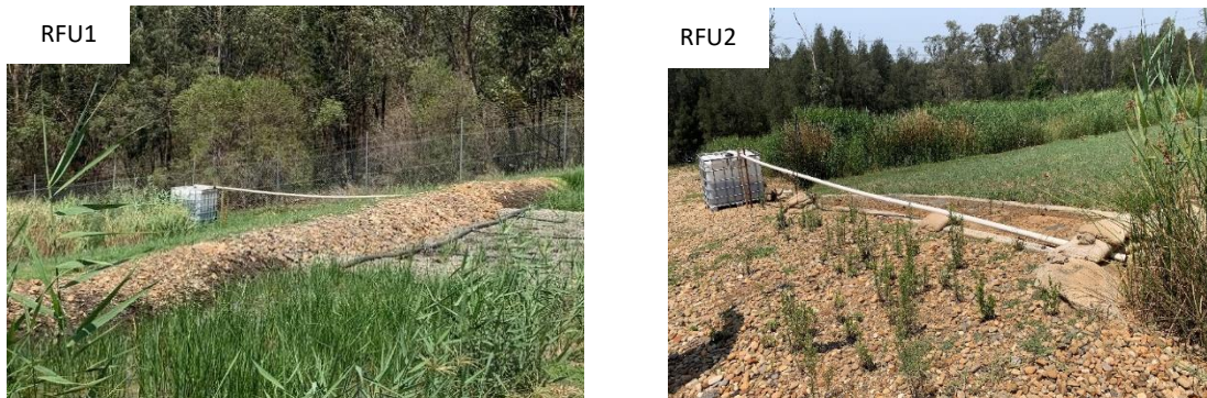
Figure 2. 2 RFUs installed on site
